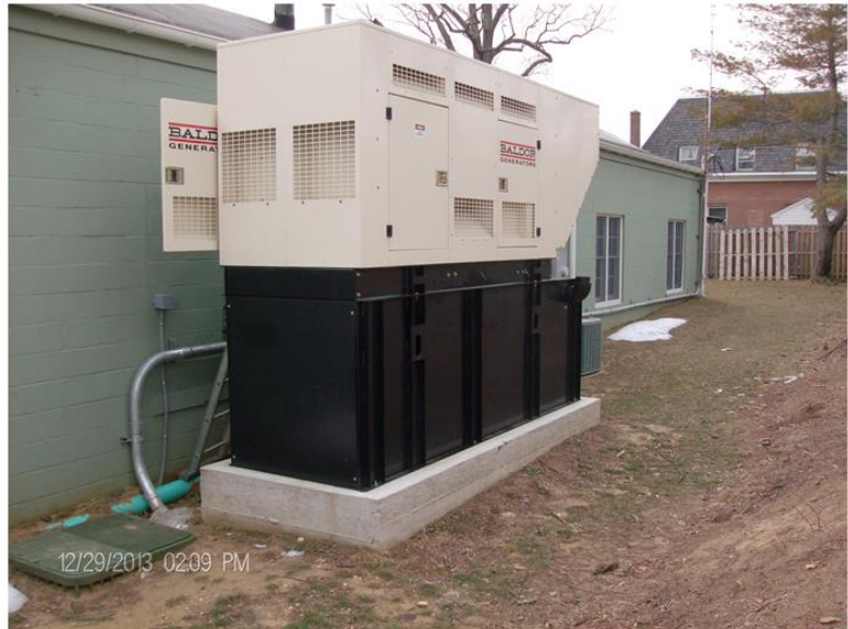
Figure 4: Emergency Generator at the DPW Yard
