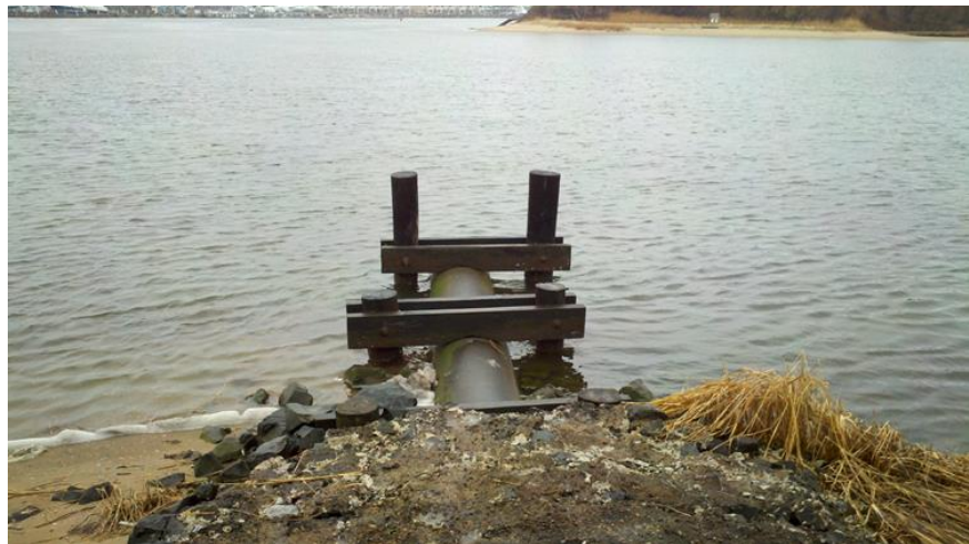
Figure 5: Waterman Avenue Stormwater Outfall
