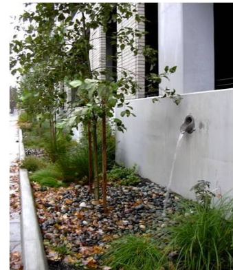
Figure 7: Downspout Disconnection (Source: EPA)
