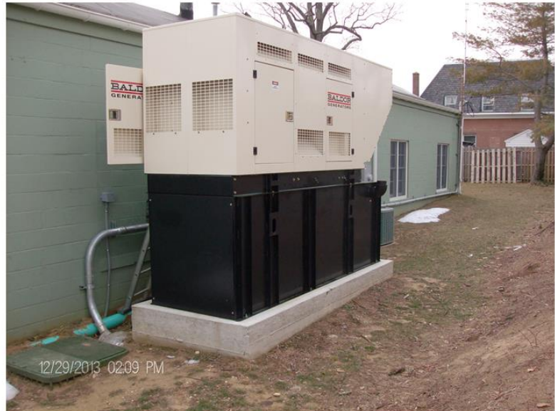
Figure 4: Emergency Generator at the DPW Yard
